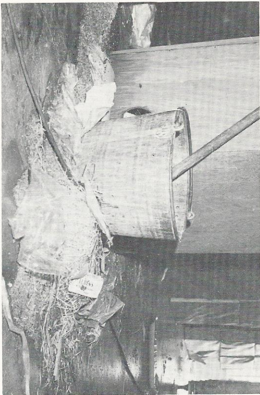
A Fire about to Happen!
