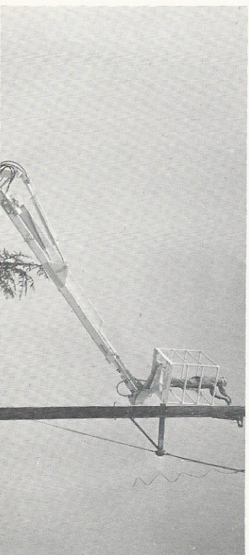
Fire Alarm Installation
